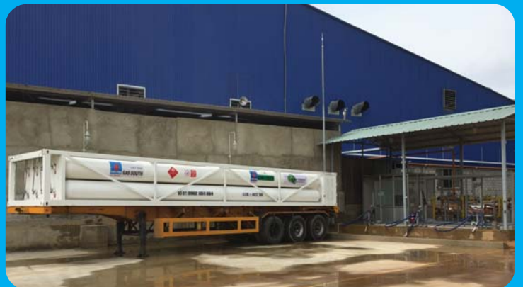
TÂN TOÀN PHÁT CERAMIC Install CNG System & Supplying CNG- PRU 1000 Sm 3 /h
