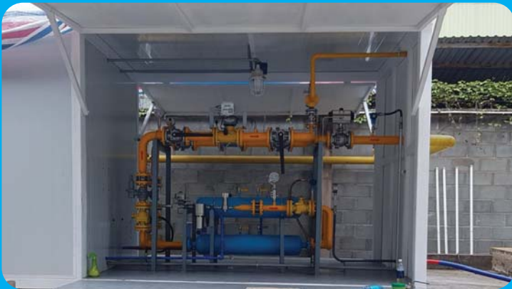
DELTA CNG STATION Install CNG Station PRU 1000 Sm 3 /h
