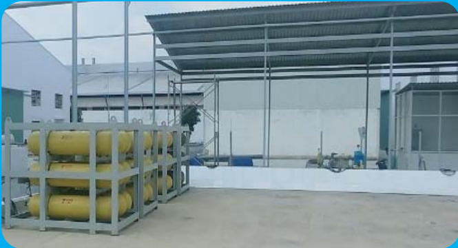
KIM PHONG WOOD Install CNG System & Supplying CNG- PRU 200 Sm 3 /h
