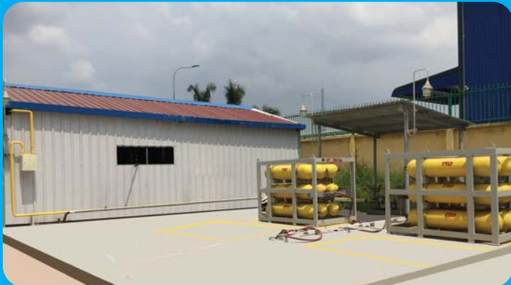
VLAND BIOTECH Install CNG System & Supplying CNG- PRU 100 Sm 3 /h
